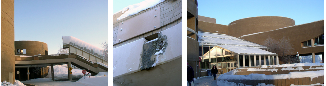
Existing Main Entry at the Second Level + Details of Existing Conditions Image Source: RIM Architect Design Team
