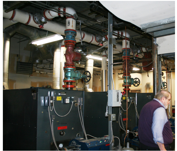
Original (1986) Boilers Image Source: RIM Architects Design Team
